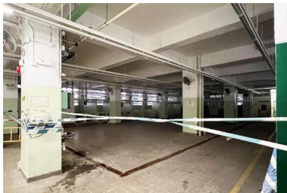
Image 12 Tang Lung Chau Market 1 st Floor closed image (Site visited at 18 October 2022)
