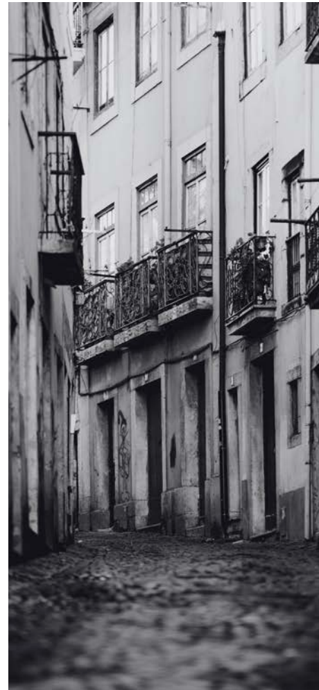
FIGURE 22: LEANING HERITAGE HOUSES IN LISBON, PORTUGAL
