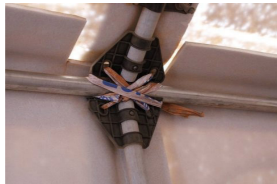
Figure 4 Dezeen. (2014). DIY repairs to the frame of a prototype Better Shelter. [image] Available at: https://www.dezeen.com/2017/04/29/united-nations-admits-10000-ikea-better-shelter-refugees-mothballed-fire-fears/ (Accessed 15 November 2023).
