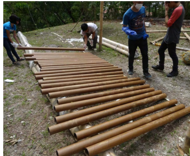
Figure 32 Shigeru Ban Architects. (2024) Process of constructing the Paper Log House. [Image] Available at: https://shigerubanarchitects.com/works/hh/houses/paper-temporary-shelter/ (Accessed 29 December 2023)
