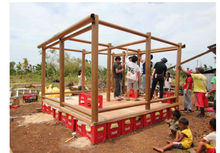
Figure 30 Shigeru Ban Architects. (2014). Construction process of the Paper Log houses in the Philippines. [Image] Available at: https://shigerubanarchitects.com/works/hh/houses/paper-temporary-shelter/ (Accessed 29 December 2023)
