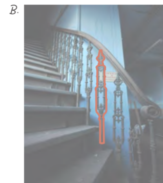
Cast iron railings. Cast iron as a material boomed in popularity in the Victorian era and more so with industrialisation to the point where decorative cast iron railings were mass-produced.
