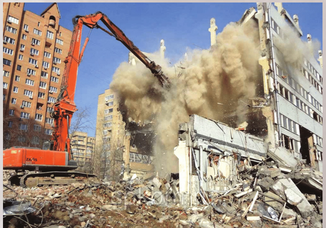
Fig.1 - demolition of a building showing the dust polluting the air and created waste
