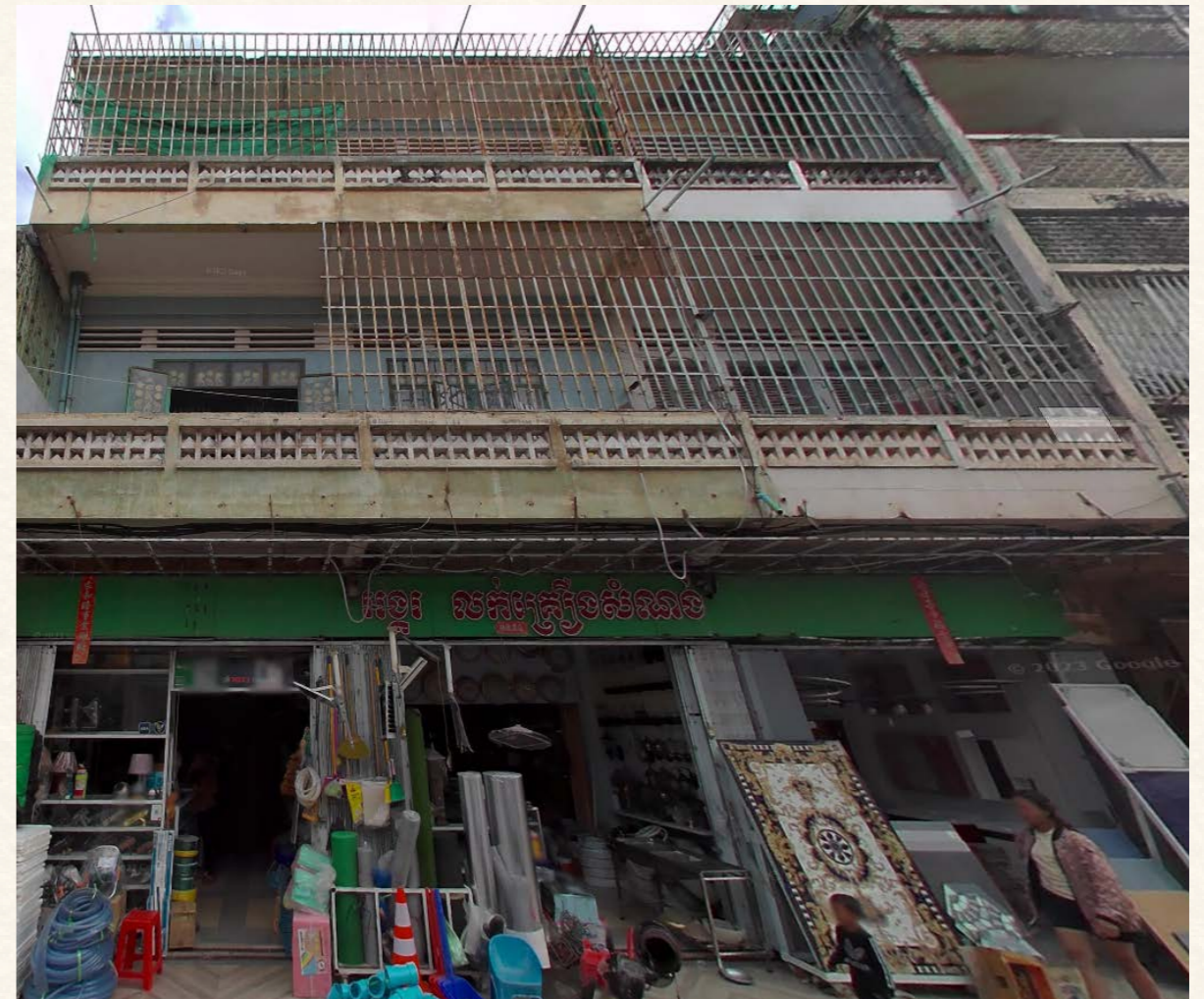
Note. Current condition of House 99's facade. From Google Maps street view [Photograph] by Google Maps, 2023.
