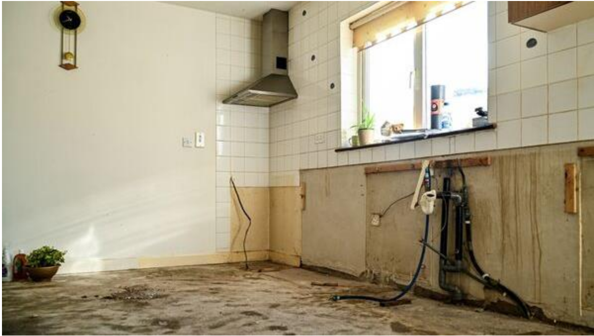
(Hoare, 2023) (Picture: Chani Anderson – Middleton home destroyed during flooding )
