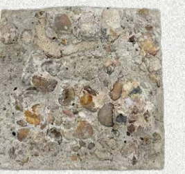
Recycled Fine + Silica - Dry and Exposed
