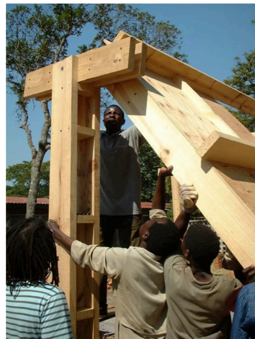
Figure 5: Community working together in Mzuzu to build the timber frame of the modular system
