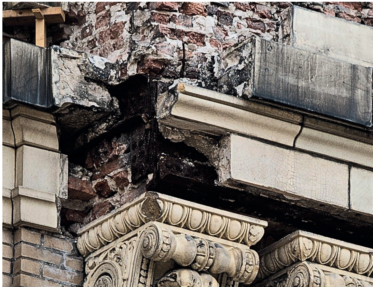
Figure 4: Exposed historic masonry and disrupted structural continuity, illustrating the ethical dilemma between aesthetic falsification through concealment and the legible articulation of a tectonic junction.
