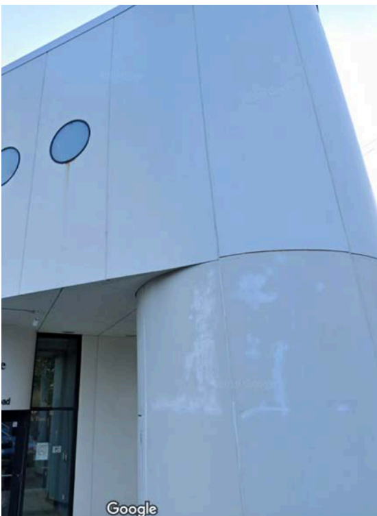
Fig. 12 Screenshot of Lakeside Bank 1055 W. Roosevelt Rd porthole window rust and damage (captured 2019)
