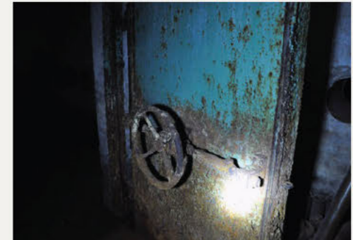
Soviet civil defence shelter - hermetic door leading to an abandoned shelter. https://loveopium.ru/arxitektura/bomboubezhishha-i-bunkery-rossii.html
