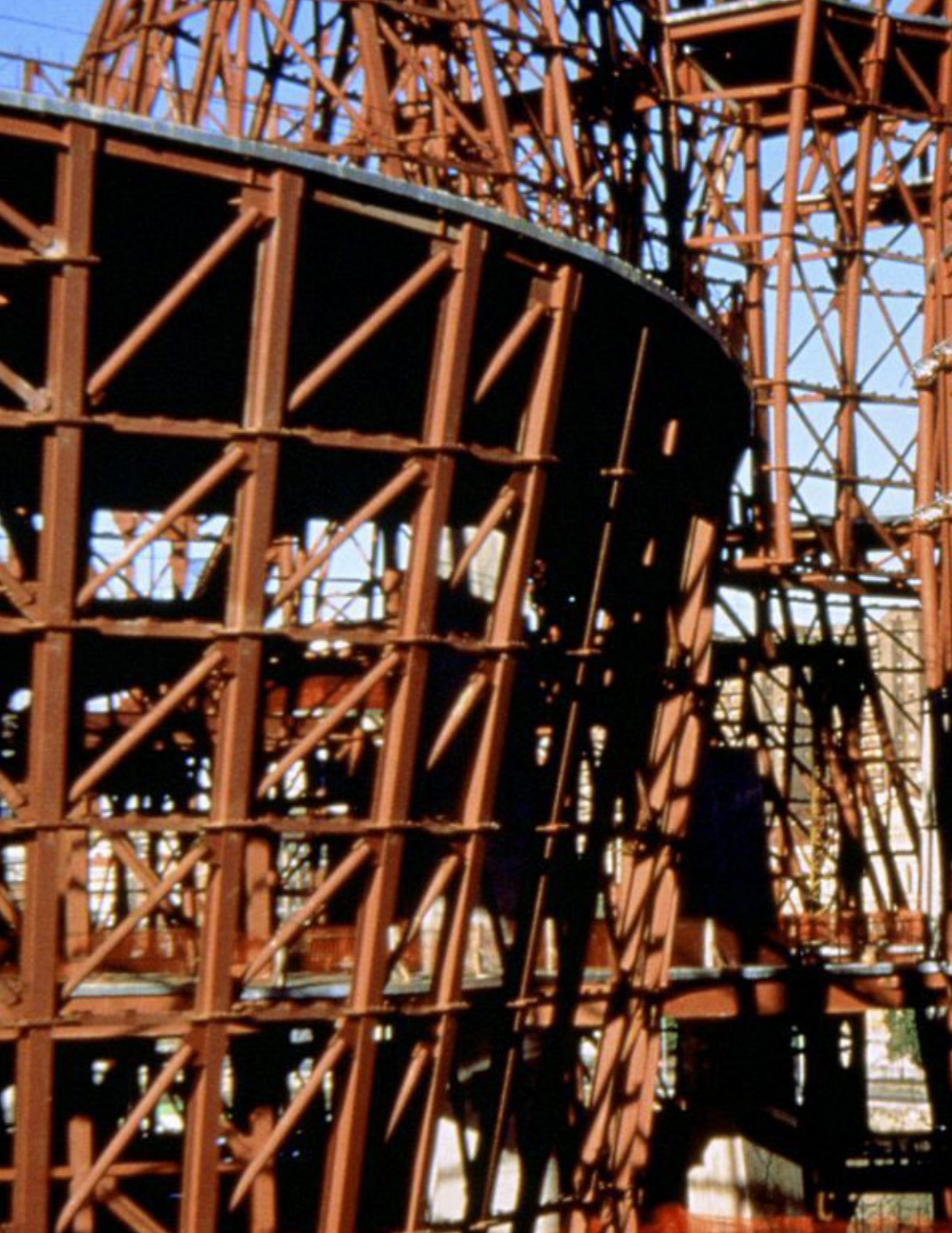
Figure 7. The Guggenheim Museum steel frame during construction before rapping the titanium on to it.
